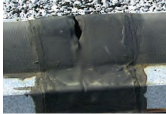
Splice Failure on Competitor's product
